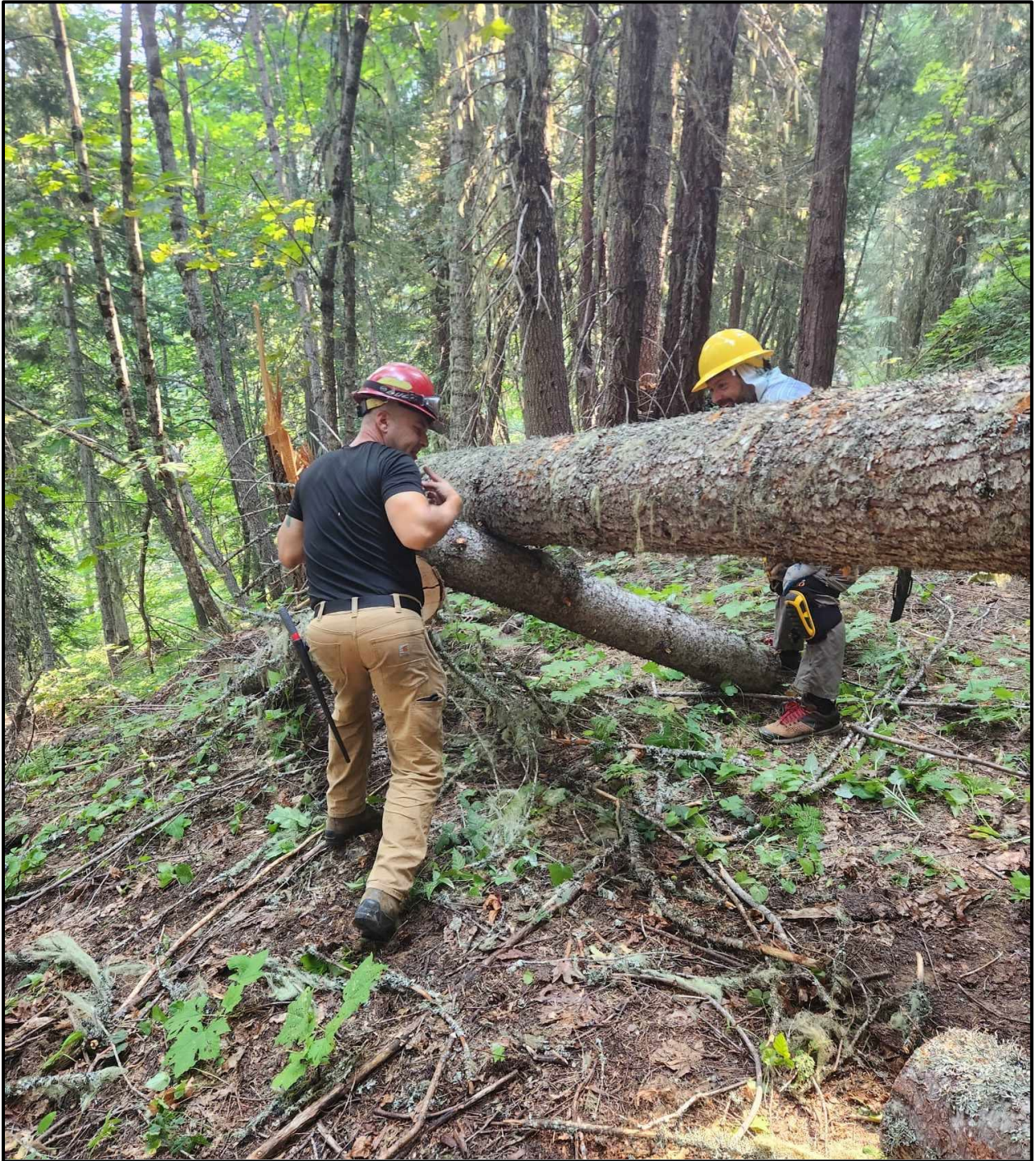
Figure 2: USDA and UTB crews work to efficiently remove a suspended log within proximity to Yellow Jacket Camp.
